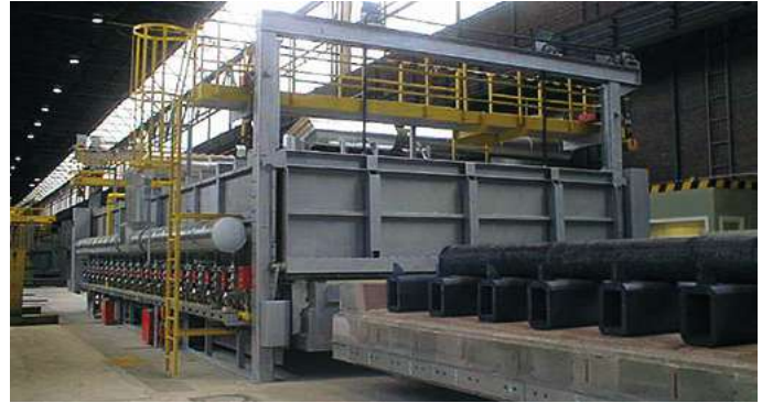
Metallurgical industry: bogie hearth furnace
